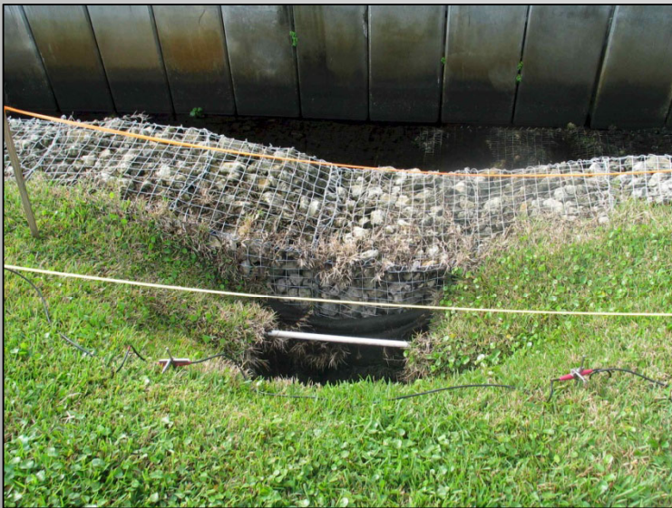
Sinkhole Collapse Feature
